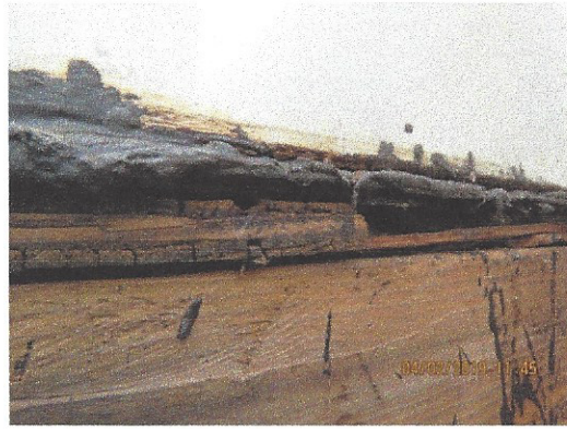
Re nailed with 8D all plywood roof deck see permit RDA 8D spaced 6" on edge and field
